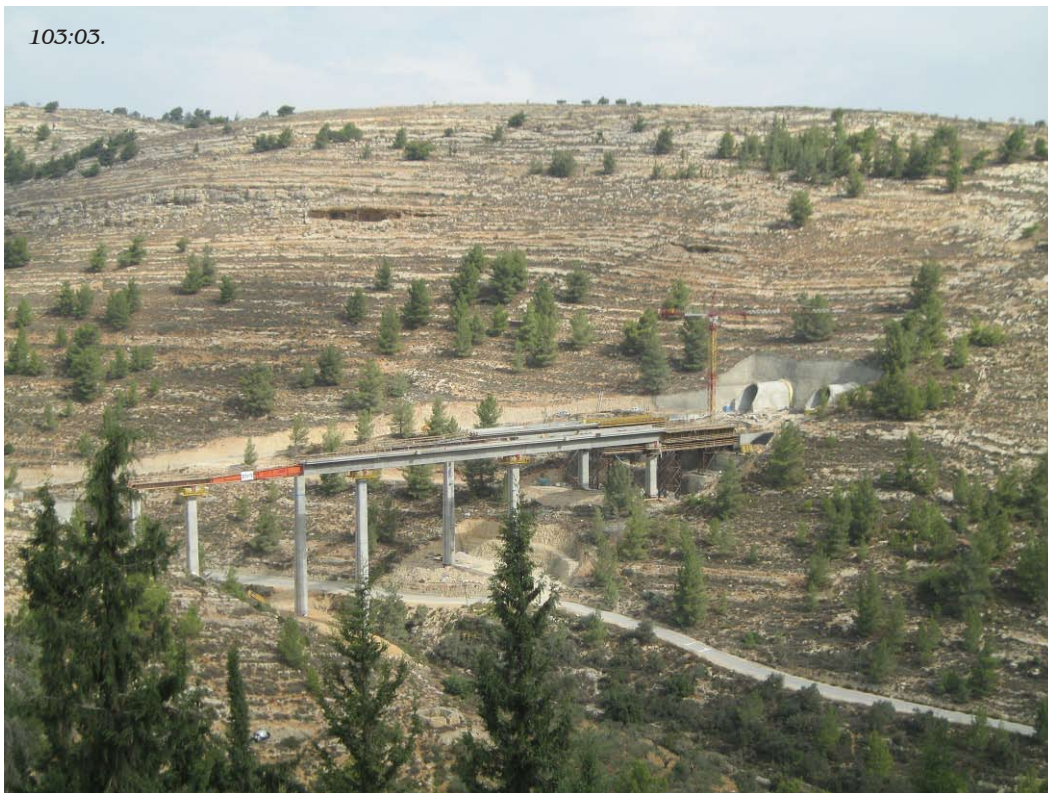
Works continue on the new Jerusalem line - here is a viaduct and tunnel near Mevasseret Zion. (Photo: Sybil Ehrlich).
