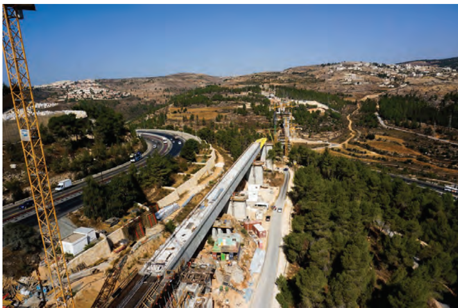
104:3 The Cedar Valley viaduct on the outskirts of Jerusalem - an aerial view (this page) and a computer-generated picture of the completed viaduct - next page. (Photos from Transport Ministry.)
