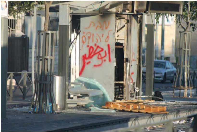
Damage caused to the Jerusalem tram stop at Shua-fat: The graffiti reads 'Death to the Jews'. (Photo by Olivia Fitoussi of CityPass, via Aahron Gazit.)
