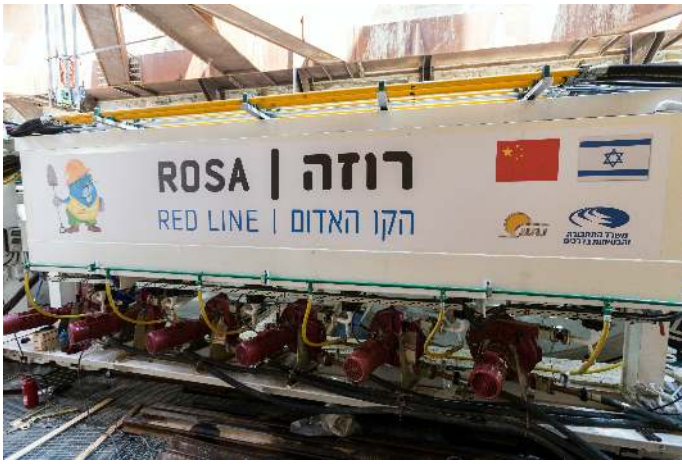
Preparatory works for extending the Red Line at Moshe Dayan St., Neve-Ya'akov.
