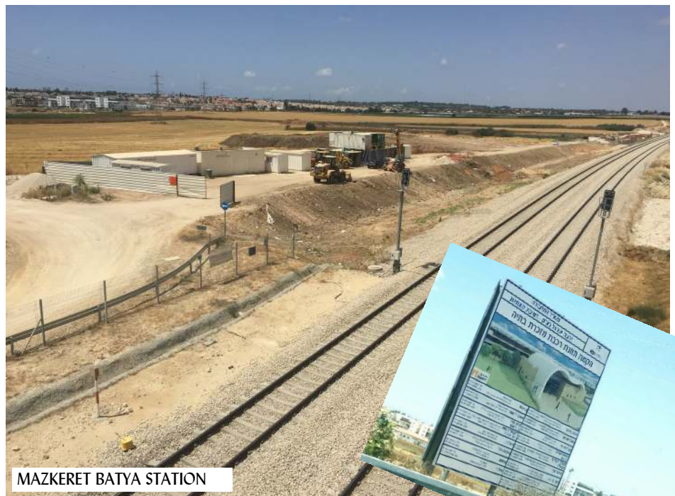
Inset: New sign for Mazkeret Station
