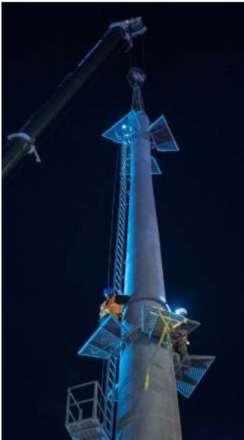
• Installing masts for the new Haifa cable car 08.04.2019. (Photo: Transport Ministry via Aharon Gazit)
