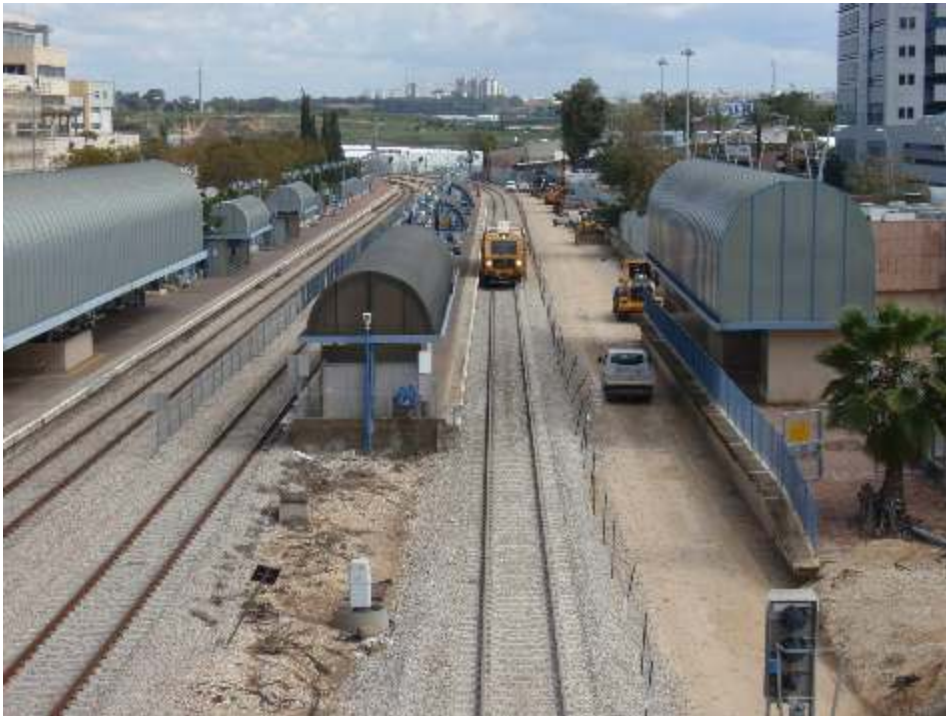
• Works under way at Rehovot station which is being rebuilt and a fourth track and platform added. The situation as at 1st. March. (Photos Aharon Gazit)
