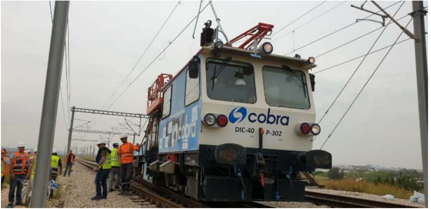
Catenary repairs on the AI Jerusalem line (photo courtesy of Matan Berkovich, IR Press office.)
