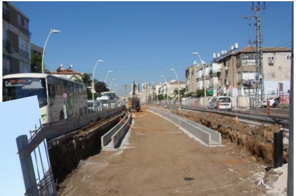
Works on the Tel-Aviv LRV/METRO Red Line in Petakh-Tikva at Jabotinsky Road.
