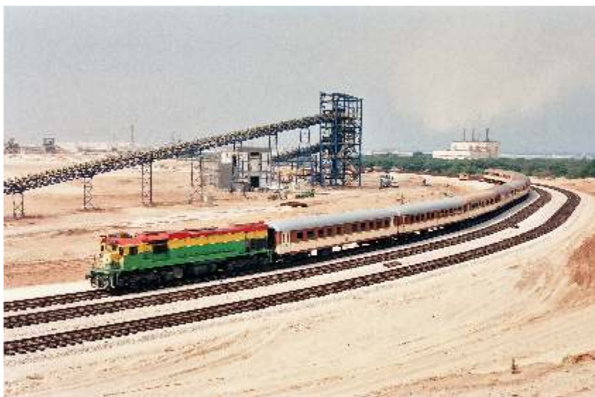
• Ashdod Coal station under construction and a special 9-coach passenger train for the Bonds headed by EMD G26CW-2 no. 612 ready to depart to Shikma Junction, 9.8.1988. • (photo: Harel Even)
