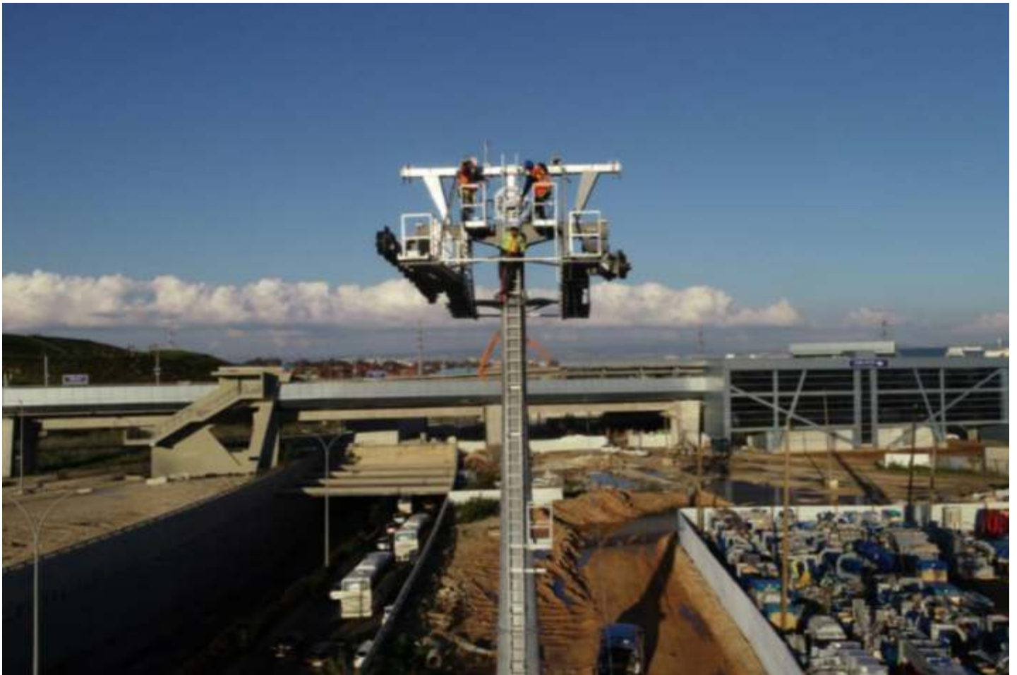
• Work on masts for the Haifa cable car (Rakbalit); provided by courtesy of Yefe-Nof.
