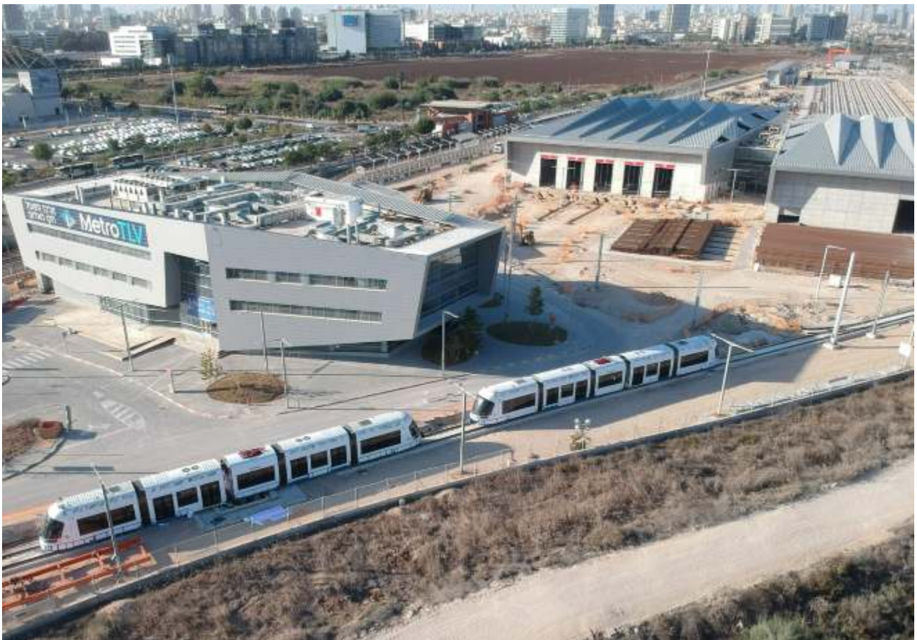
• The Red Line depot at Petach Tikva under construction and the first train sets. (Photo Gilad Furst)
