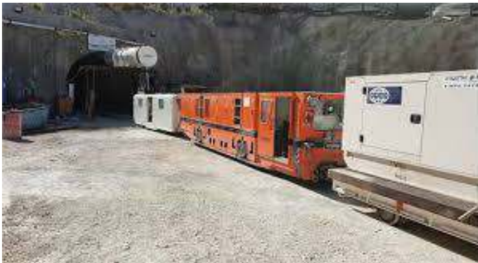
136:03 60CM GAUGE LINE FOR MEKOROT BUILDING A 33KM WATER TUNNEL TO JERUSALEM FOR THE HAGIHON COMPANY
