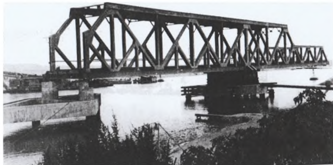
25:18. The bridge over the Suez Canal at El Ferdan, after it had been damaged by a Dutch cargo vessel. 1947. (D.S. Currie).
