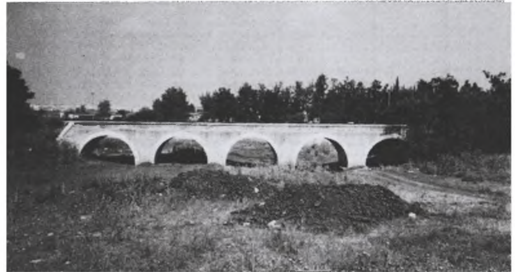
The first bridge north of Ras el Ain (Rosh Ha' Ayin) station, as seen from the east in May 1993. Photo: Alon Siton.
