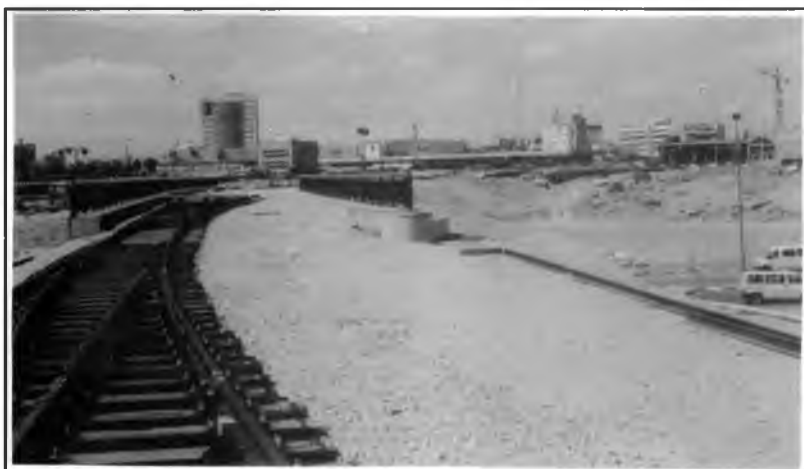
View from the railhead by the road viaduct at entrance to new Beer Sheba Central station, 13/3/2000. The crane at Right marks the new building under construction; the low flat roof in the middle of the picture is the Bus Station
