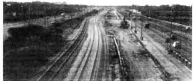
The site for the junction for the new line to Ben Gurion airport (and eventually Modi'in and Jerusalem) - the two existing tracks in the median strip of the motorway have been slewed to make space for the new junction. View towards Tel Aviv. Jan. 2002.
