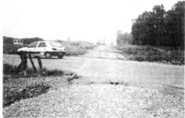
Earthworks at a road crossing near Na'an on the Jerusalem line. April 2002.
