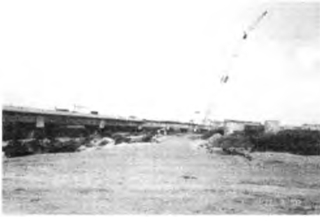
The line to Ben-Gurion airport is taking shape. Seen here is a large bridge over the Ayalon river not far from the airport.
