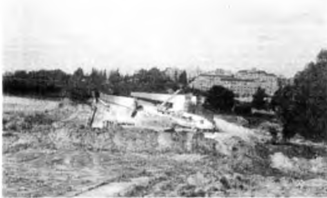
Kfar Sava (Nordau) station under construction, looking towards the new Sokolow station.
