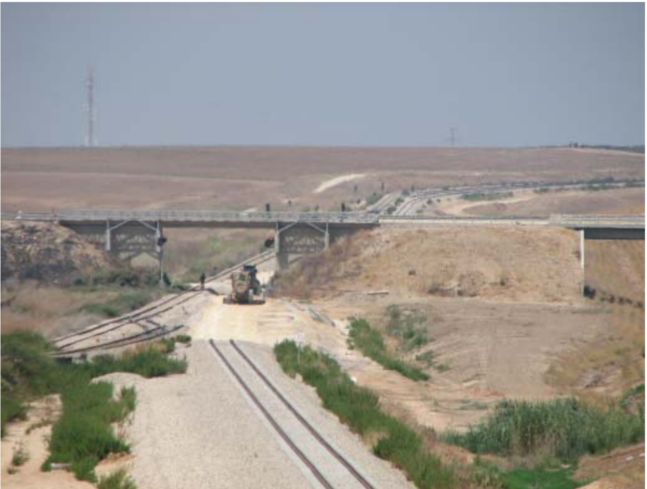
The new section on the line to Beer-Sheva near Kfar-Menakhem replacing the old one on the left (already dismantled); photo by Aharon Gazit (79:04a)
