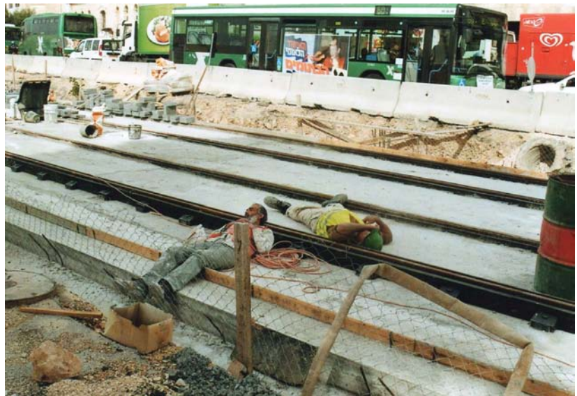
84:03/1 "Not a terrorist attack, but "men at work" on the tramway on Jaffa Road, Jerusalem, Feb 09
