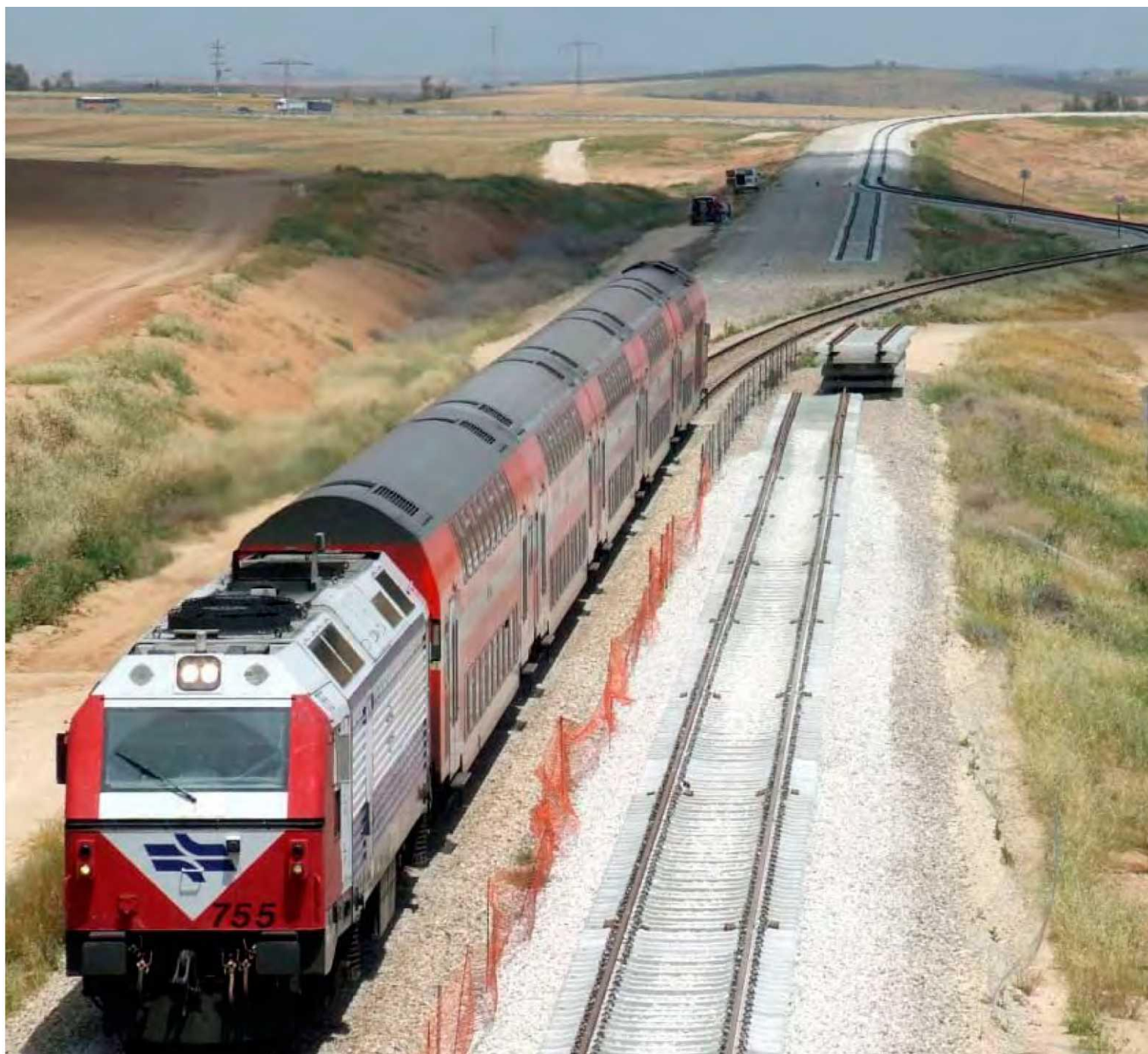
87:01. . 755 hauls five Gornitz-built double-deck coaches through track works between Tel-Aviv and Beer-Sheva near Kfar-Menakhem; the new double-track and less sharply-curved alignment is almost ready for connection. (Photo courtesy of Shazar Wiessman, IR Spokesman).
